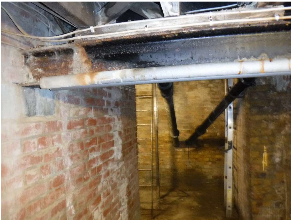
Photograph 005 – View of steel I beam running onto padstones within wall in Area B
