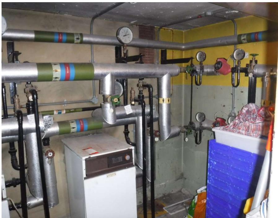
Photograph 017 – General view of boiler room at rear of Area J
